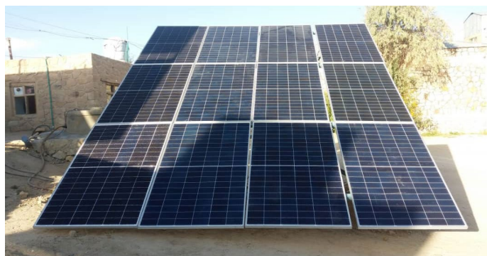
WHO provided solar power system for water supply network in Azro CHC in Ghazni province.
