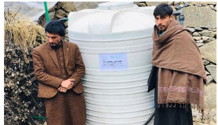
Installation of water tank at Shamash (Sohil Tangi BHC) water supply extension and tank installation at Kareen SHC, Kunar.
