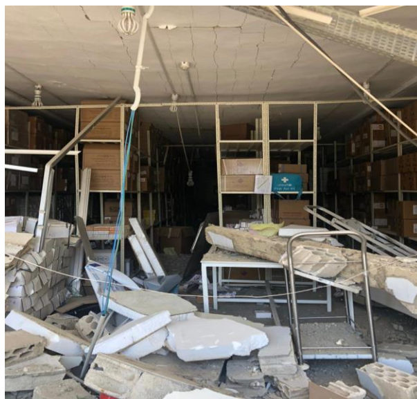
Heavily damaged central drug warehouse, WHO Lebanon
