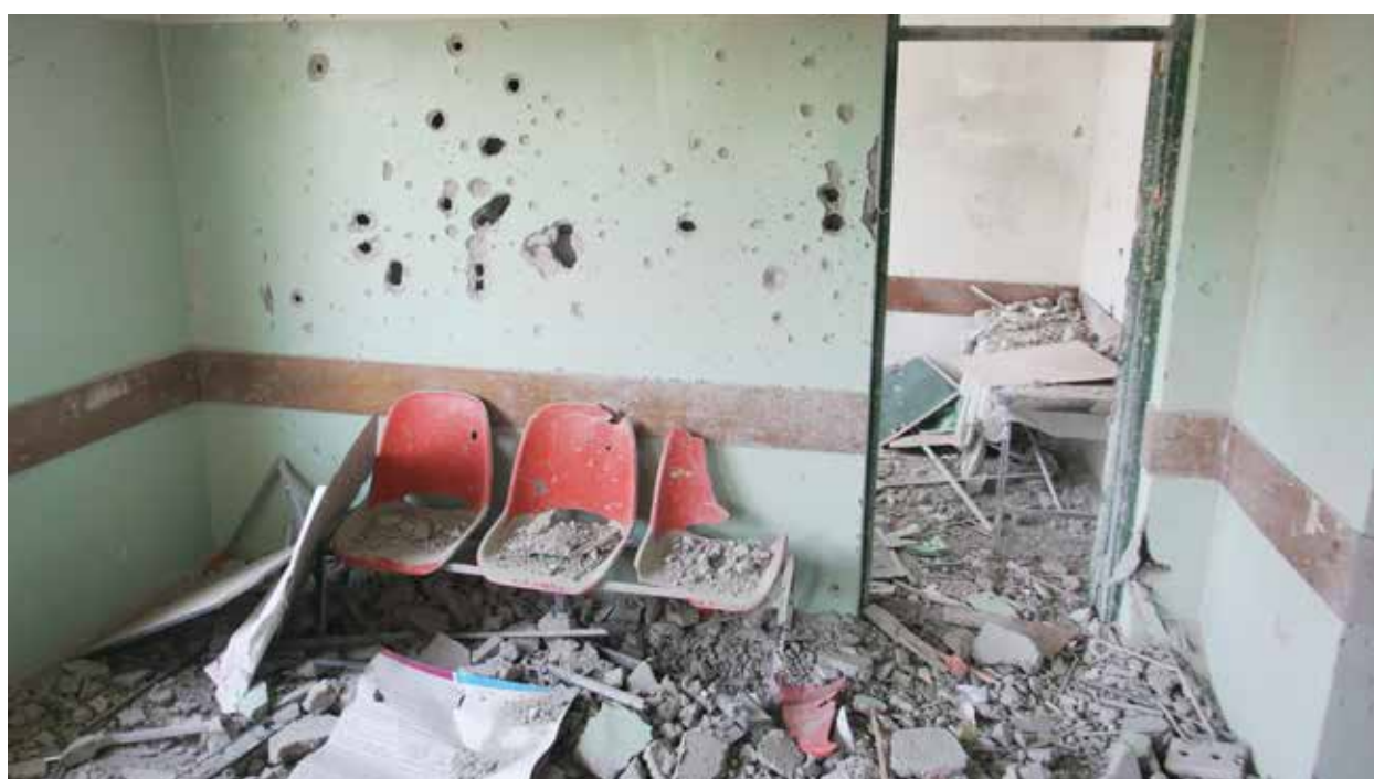
Al-Quba primary health care center which was destroyed in 2014 summer war © MoH
