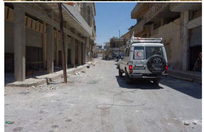
Al-Qusair's only hospital has been destroyed hospital (top);
